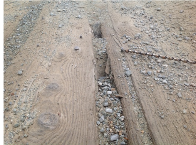
nails starting to protrude
